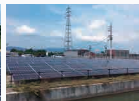
Wakayama Solar Power Plant
