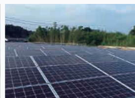
Kagoshima Solar Power Plant
